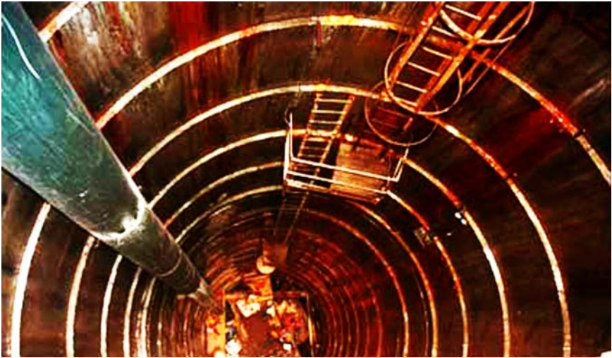
Figure 4.19(a). Provision of adequate artificial ventilation through a duct. Note the staircase on the right.
