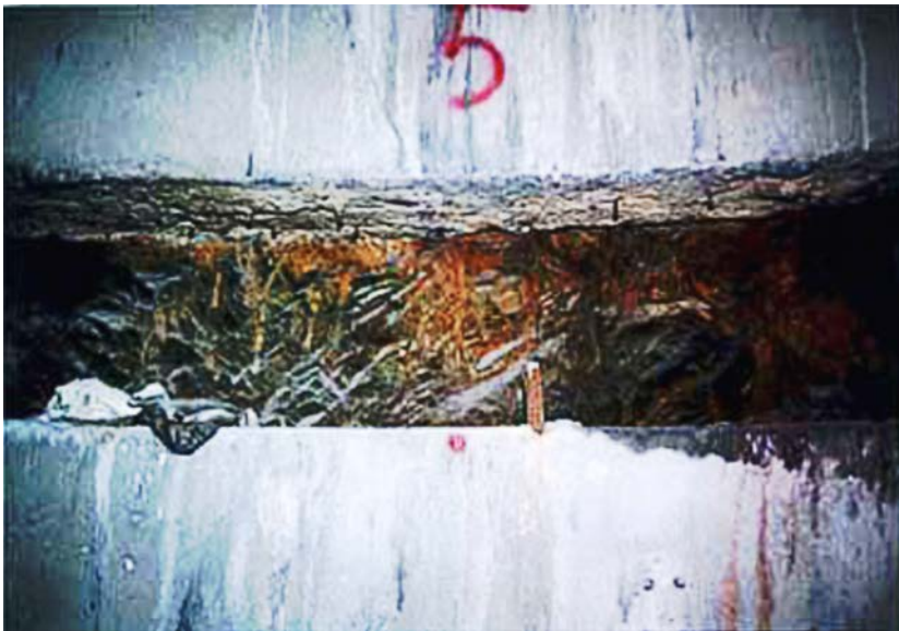
Figure 4.17(b). A closer view of the gap. Note the pins and starter bars.
