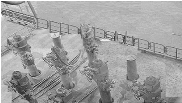
Figure 2.4. Production platform christmas tree and wellhead assembly
