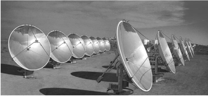
Fig. 1.14. Field of PV parabolic dishes manufactured by Solar Systems in White Cliffs, NSW (Australia). Each dish focuses the light on a compact actively cooled receiver, whose surface is a parquet of BPC cells. Each disk is rated 25 kW p nominal
