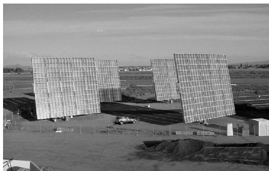
Fig. 1.13. Two-axes tracking arrays from AMONIX, installed at Arizona Public Service, Scottsdale. They use 27% efficient BPC solar cells operating at 250 \times under point focusing laminated Fresnel lenses: the nominal array power is 25 kW. This technology was licensed to GUASCOR-FOTON (Spain) in 2005 and is currently being commercialized
